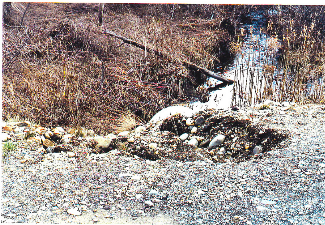
Poorly Maintained Culvert
